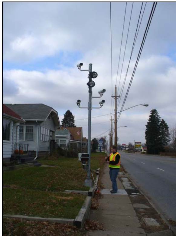
Figure 89. Davenport RLR and Automated Speed Camera System.
