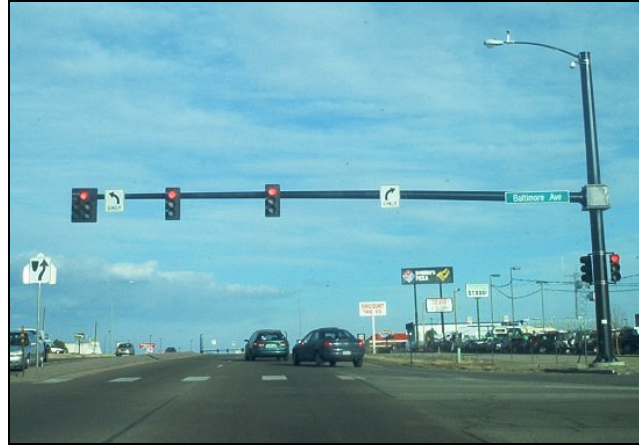
Figure 3. CDOT specified high-speed intersection traffic signal (25).
